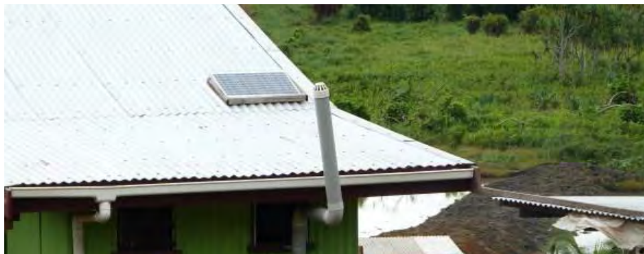
Figure 13. Solar panel in Kenani
