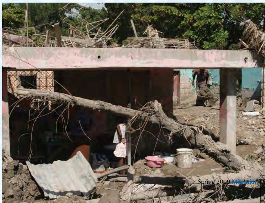
▼ The damage to Gerdine and Gerda Joseph's home is so extensive that the sisters cannot rebuild it on their own. © IOM 2008 - MHT0227 (Photo: Patrice Dougé)
