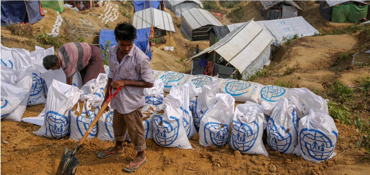
Rohingya refugees employed by IOM through a cash-for-work scheme reinforced a slope in Balukhali Rohingya refugee settlement, Bangladesh. © IOM 2018/Olivia HEADON
