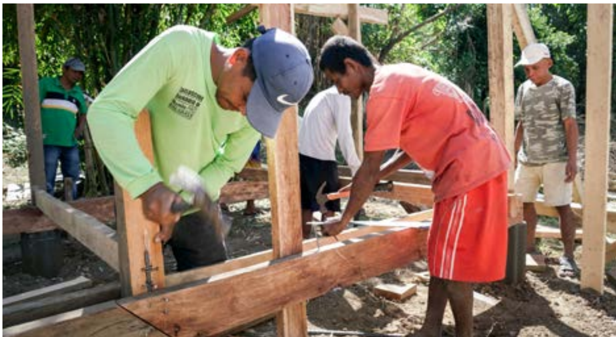
Joey (in red) helping out in the construction of his temporary shelter provided by IOM. © IOM 2019
