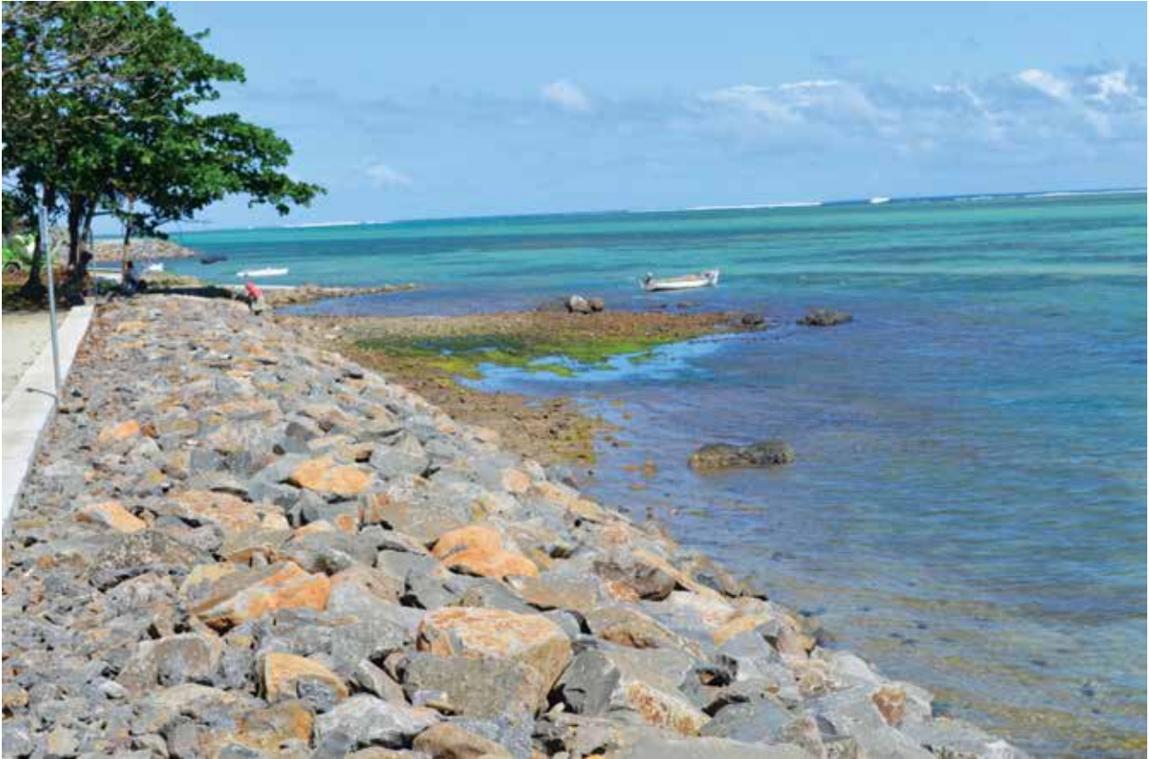
Rock revetment in the south-west of Mauritius. © Ministry of Environment of the Government of Mauritius, 2015.
