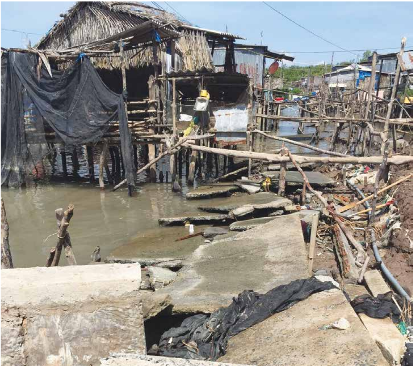
Houses and roads now stand in the water as the land erodes on the coast in the Mekong Delta region of Viet Nam.
