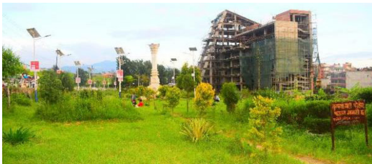
Figure 7. A building under construction in the vicinity of the open space at airport Central Dojo in the eastern side of Kathmandu Valley, near TIA
