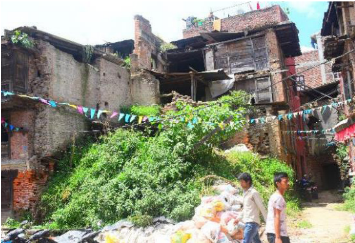
Figure 149. A damaged building in the vicinity of Talako
