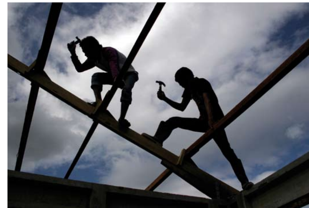
Workers on the second phase of house building at the IOM housing development at Cot Paya in Banda Aceh.
