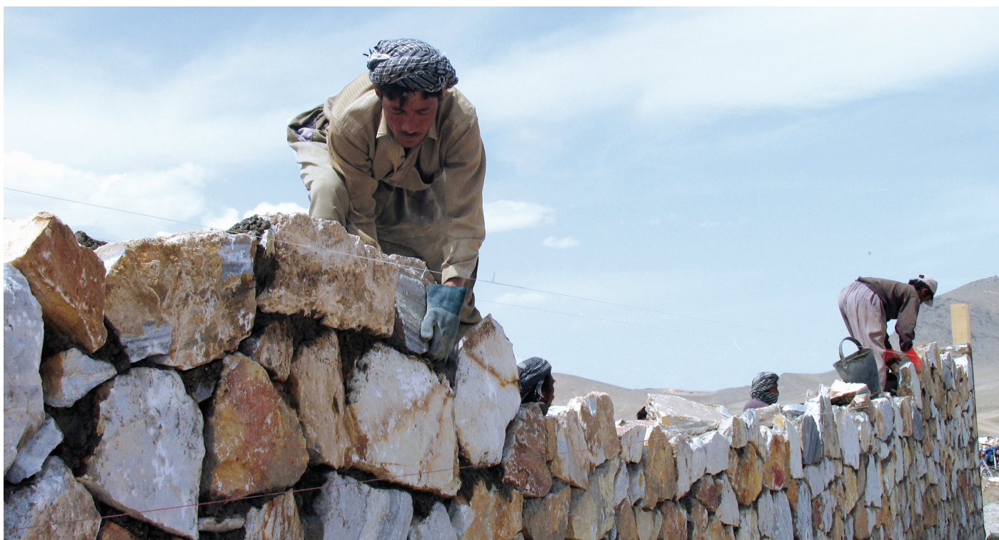
IOM begins construction work on the main section of the new Ghazni Hospital, Afghanistan. © IOM 2007 - MAF0258 (Photo: Katsui Kaya)
