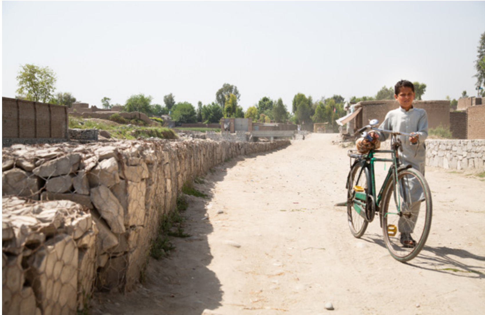
A young boy is pushing his bicycle on a road alongside a flood protection wall constructed by IOM in Nangarhar province. So far, IOM has implemented 74 disaster risk reduction infrastructure projects in 25 provinces with a total length of 15,673 meters protecting over 119 villages, 25,777 acres of agricultural land, 19,915 houses benefiting around 51,200 families, and temporarily employing over 140,000 skilled and unskilled workers. © IOM / Eva Schwoerer
