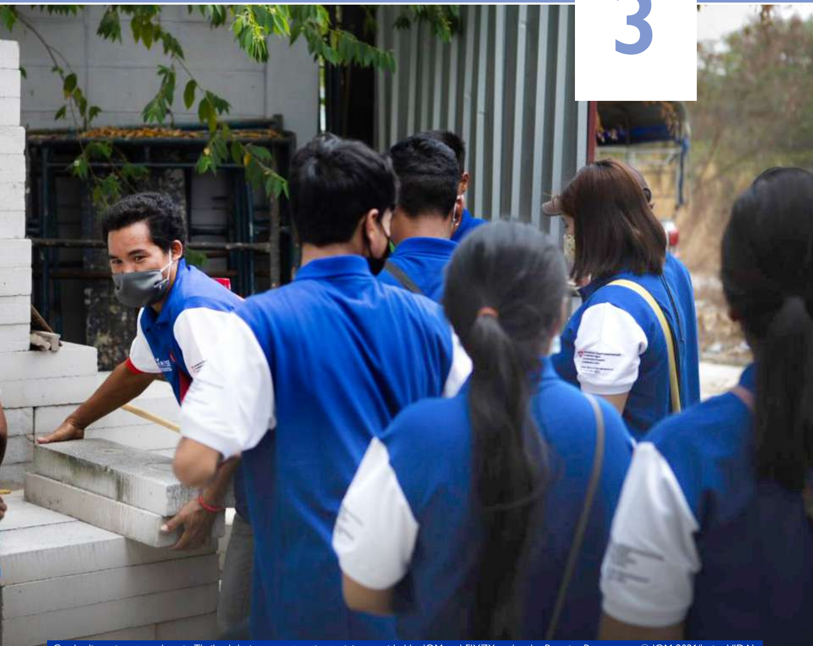
Cambodian migrant workers in Thailand during a construction training provided by IOM and FIXZY under the Promise Programme. © IOM 2021/Javier VIDAL
